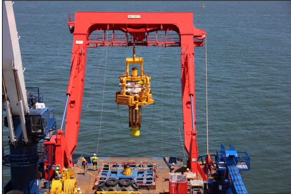
Figure 18: Deploying a Capping Stack onto the Blowout Preventer on the Seafloor (Credit: Oil Spill Response Limited)
